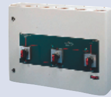
External Service By-pass Panel
